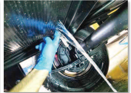
Liaqat takes a picture of himself pulling back a unit's underbelly panel showing a water leak.
